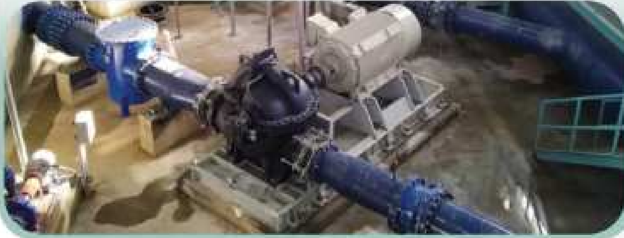
GILAN WATER TREATMENT PLANT
