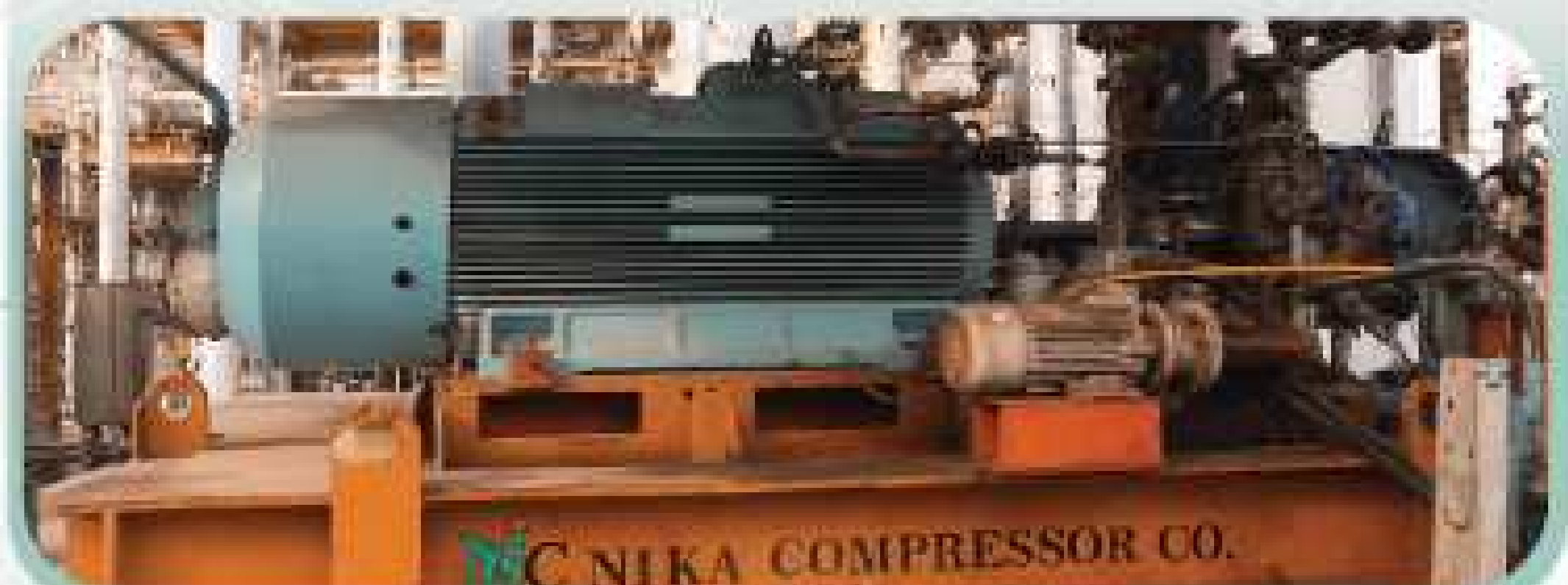
NIKA COMPRESSOR FOR 7th REFINERY OF SPGC
